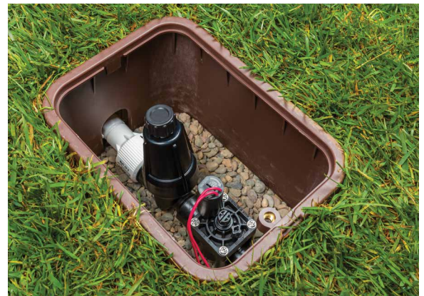
PCZ-101 installed in a Multi-Purpose Box
